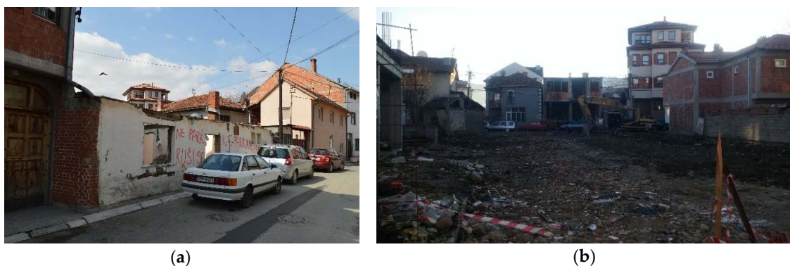
Figure 6. A cleared site for the construction of a multi-story building in the immediate vicinity of the historic center in the 7th of July Street (a) street view; (b) view of the lot.
